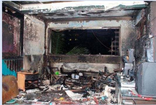
Fire and smoke damages sustained in the living room
