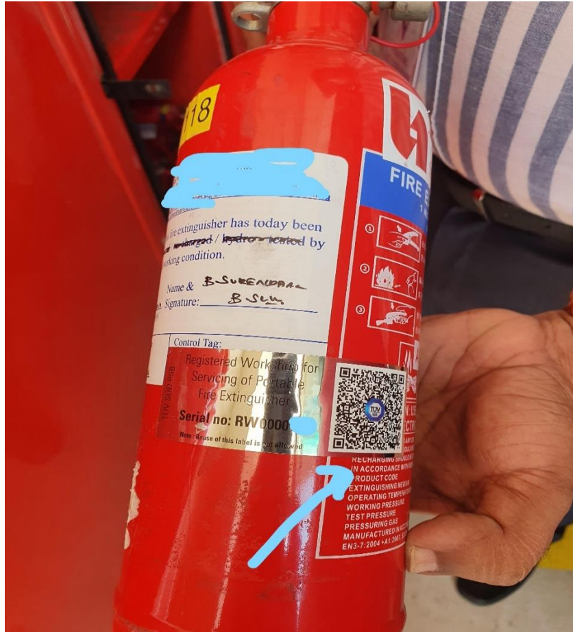
COVERING THE INSTRUCTION PRINTED ON THE EXTINGUISHER
