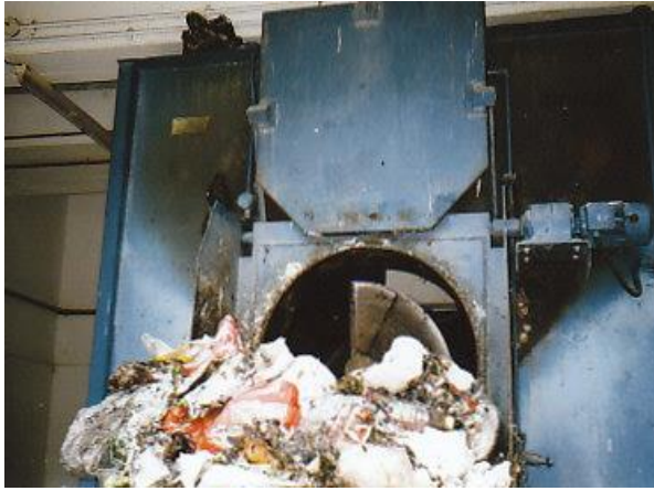
Figure 15. The RHE sustained heat damage
