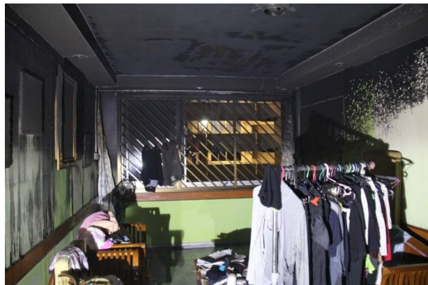
Figure 19. Other parts of the unit sustained heat and smoke damage
