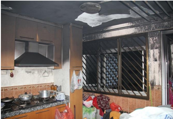
Figure 20. Other parts of the unit sustained heat and smoke damage
