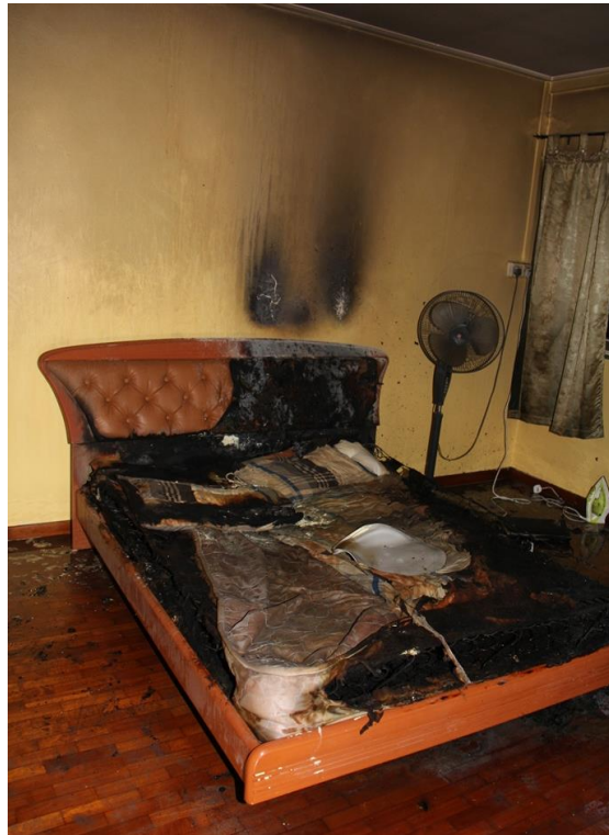
Figure 22. As a result of the fire, the bed was damaged. The walls and flooring in the room sustained heat and smoke damage
