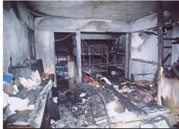
Figure 11. The fire consumed the wooden partition and spread into the living room
