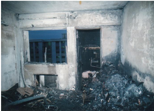
Figure 8. The entire master bedroom was gutted by fire
