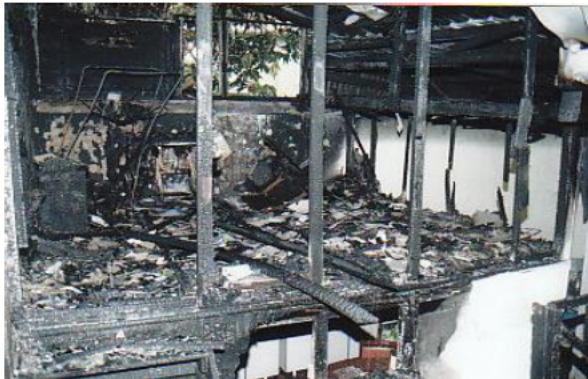
Figure 12. Fire developed and burned into the rooms
