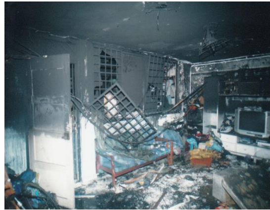
Figure 9. Other parts of the unit sustained severe heat and smoke damage
