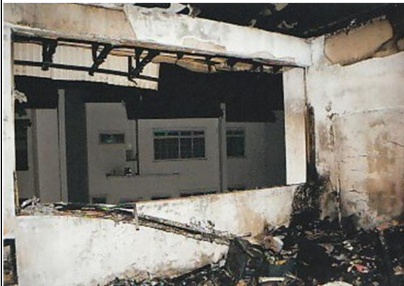
Figure 14. Fire damage was severe in the master bedroom
