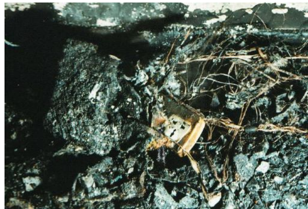
Figure 15. The burned remains of a portable socket outlet
